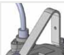
Power cable Insulation treatment. No water leaking.
